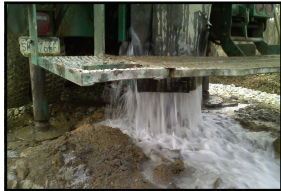
Flowing artesian well, producing 200+ gallons per minute.
